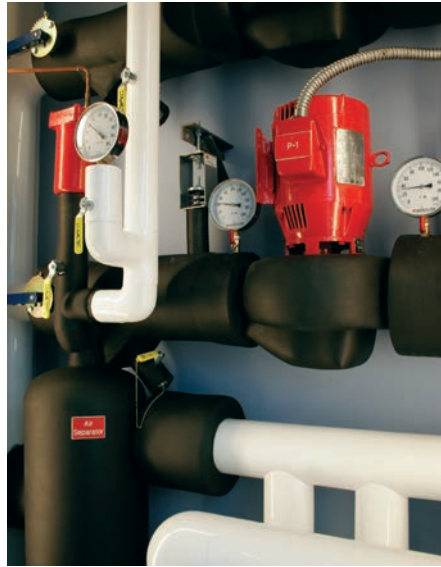
The differential pressure setpoint for the geothermal closed loop was initially set at 20 psi via hand calculations. Through trial and error, the final setpoint was lowered to 15 psi.
