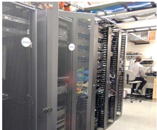
Virtualized servers reduced server footprint by 80%, emptying one rack entirely.
